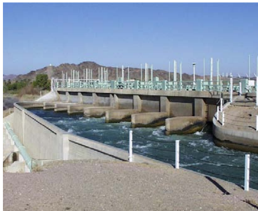
Gila Gravity Canal Headworks; 2,200 cfs max flow; 14 feet head; 2.4 to 5.9 MW potential
